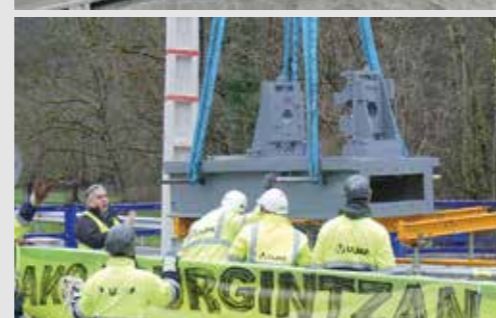
>> Sequence of images that show the process that was followed for disassembling the machine at the installations of ULMA Construction in Garibai, until its final placement in the roundabout.
